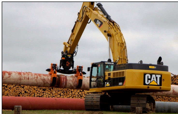
The DECKHAND “L” lifting a 36” pipe on an excavator provided by Pipeline Machinery International.
